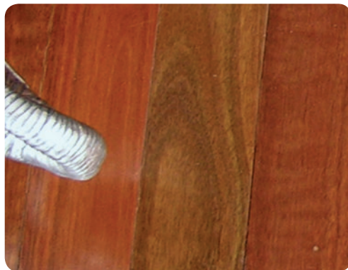
The nail penetration is to the bottom right of the photo.
