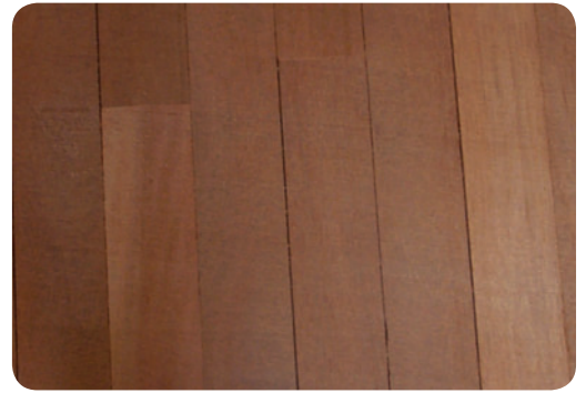
Wide gaps due to high moisture contents at the time of machining.
