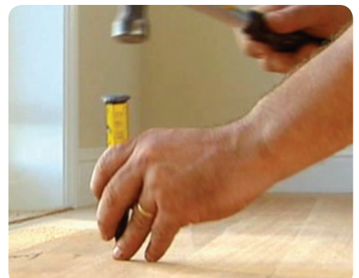
Nails to be punched and holes filled.
