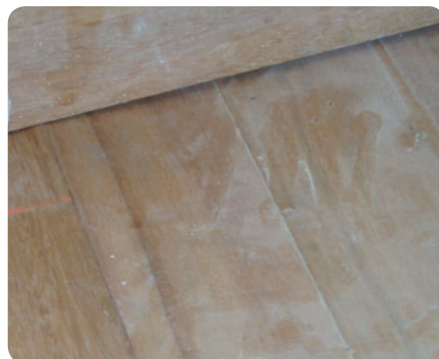
Prior to sanding, the floor should be assessed to ensure that it is in a condition suitable for sanding.
