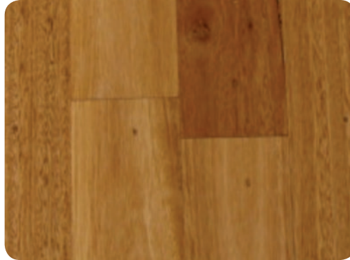
Boards ends should be spaced out and preferably 450 mm or more apart.
