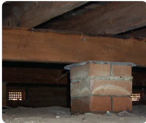
A dry sub-floor space and adequate ventilation is essential for good floor performance.
