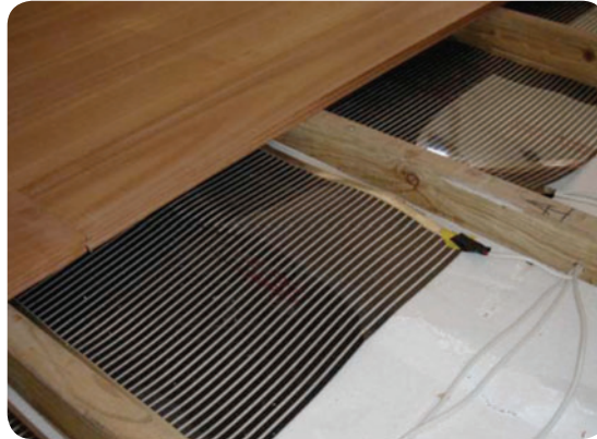
Blackbutt flooring (130 mm wide) with electric underfloor heating in Adelaide.
