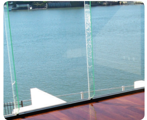
Greater localised shrinkage and possibly some cupping can be expected with high sun exposure.
